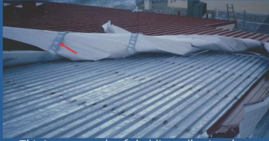
This is an example of cladding adhesion that was not tested. (and the membrane was not installed correctly.)
